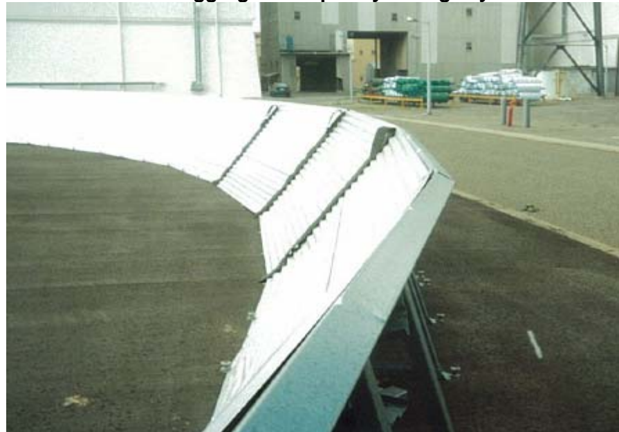
Plate 1: Sand and aggregate temporary storage system
