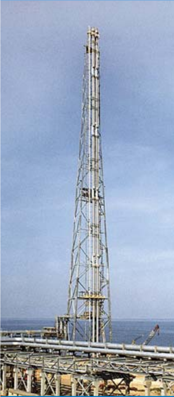
Plate 6-4: Typical Flare Tower
