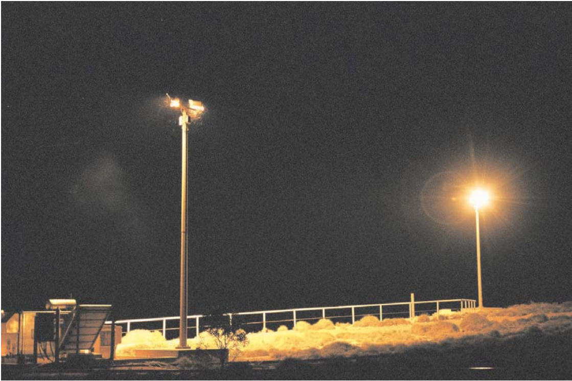
Plate 6: 400W sodium vapour lights at the Landing
