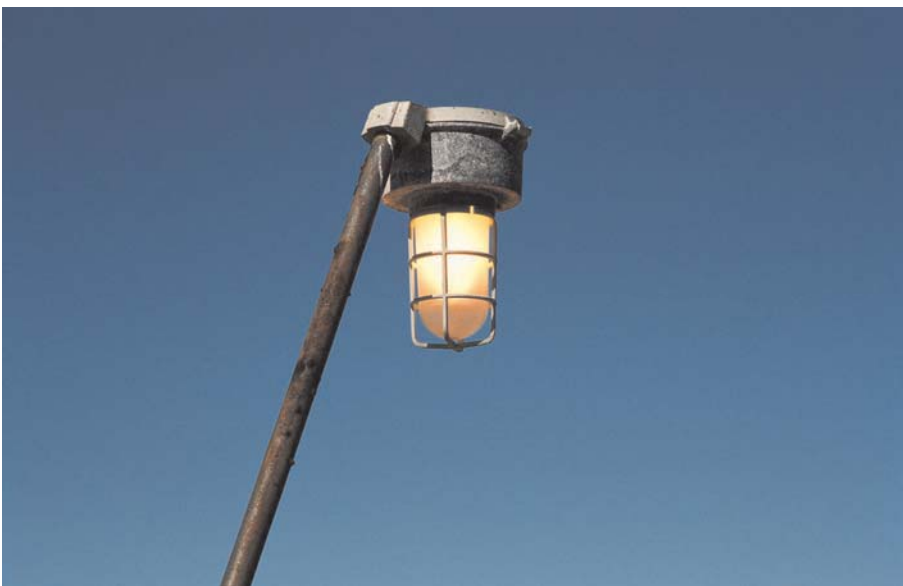
Plate 9: 40W sodium vapour light at the suck back pump, close up
