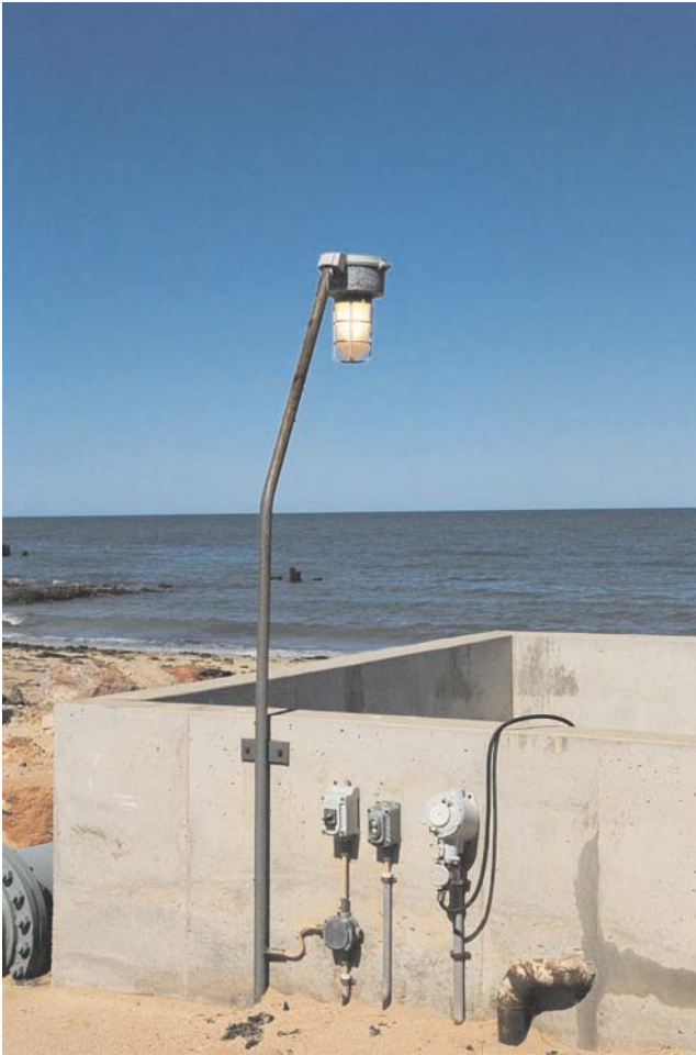
Plate 8: 40W sodium vapour light at the suck back pump
